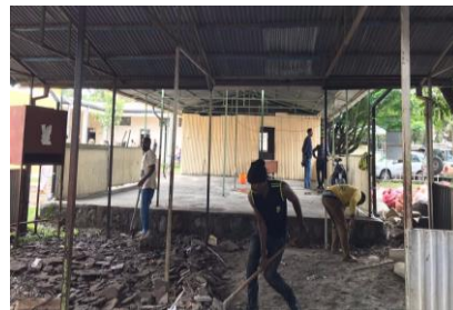
Waiting room being built with support from the Community after scorecard feedback
